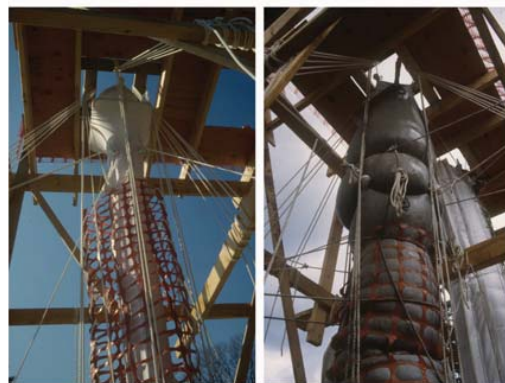
8. Fabric-formed (Spandex) concrete column, before and after pouring concrete. Bar Harbor, Maine. 1990
